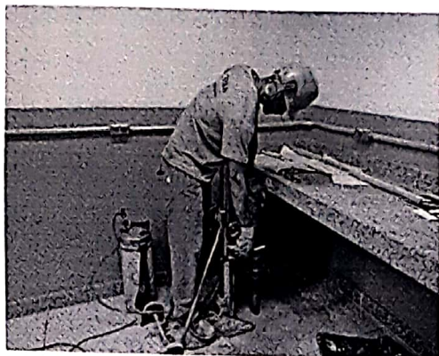
Furos no concreto
